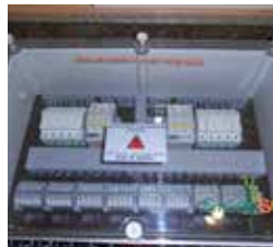
Solar Array Junction Boxes
