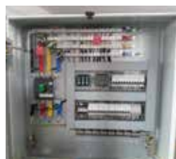
AC Distribution boards - 1-500 Kw
