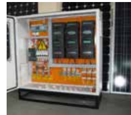
RTU - Telecom Panels
