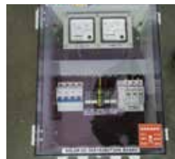
DC Distribution boards - 1-100 Kw
