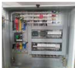
AC Distribution boards - 1-500 Kw
